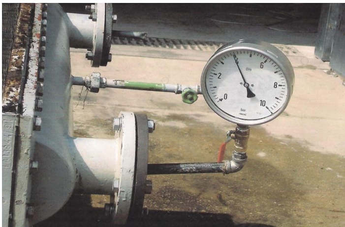
Figure 1: Radiator Pressure Test Experimental Setup (at Shiroro Power Station)
