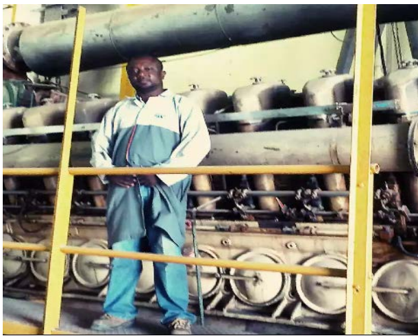
Figure 3:A 3MVA 11kV Generator's Prime Mover: Metallic Barriers are Painted Yellow [10]
