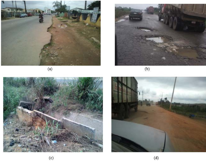
Fig 1.0: Some common Failure types along Nigerian roads a. Edge Failure along road in Bodija, Ibadan b. Cracks and Potholes along Port Harcourt road (Source: Aliyu, 2014) c. Failed Drainage along Lagos road (Source: Agbonkhese et al, 2013) d. Asphalt surface failure along Atan Ota – Lusada – Agbara Rd, Ogun State
