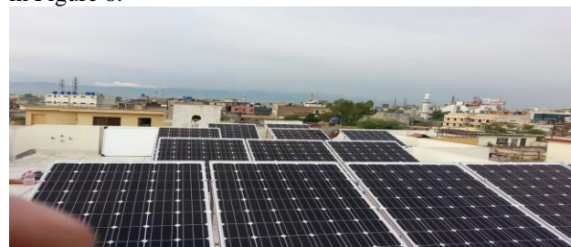
Figure 8: Solar panels install domestically in Pakistan.
