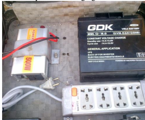
Fig. 6. PCB showing the Power Inverter and DC Battery
